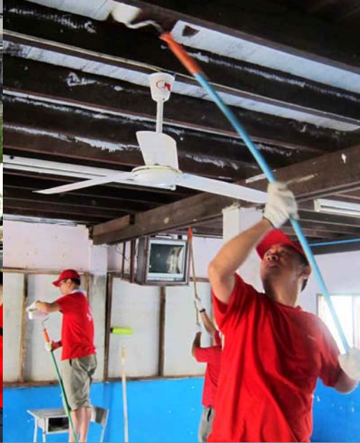
SingTel staff volunteers refurbishing an elementary school in Ayutthaya, Thailand, that was damaged by flooding
