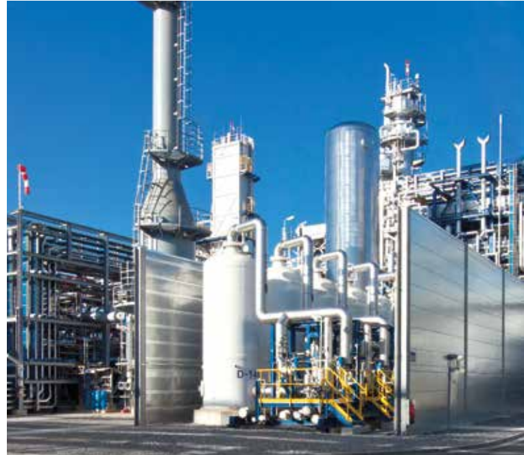
Dormagen , state-of-the-art Steam Methane Reformer unit.
