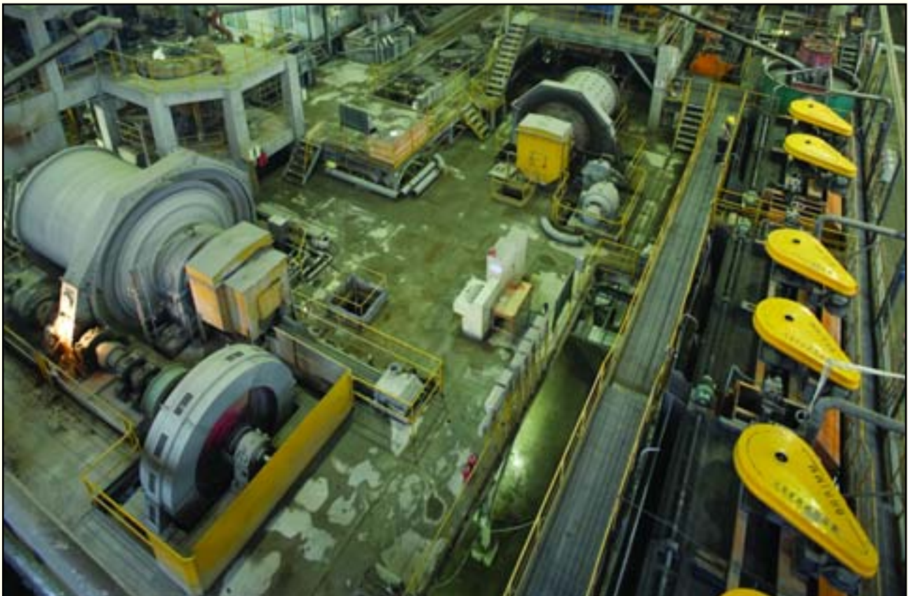
CAIJIAYING PROCESSING PLANT WITH NEW FLOTATION CELLS
