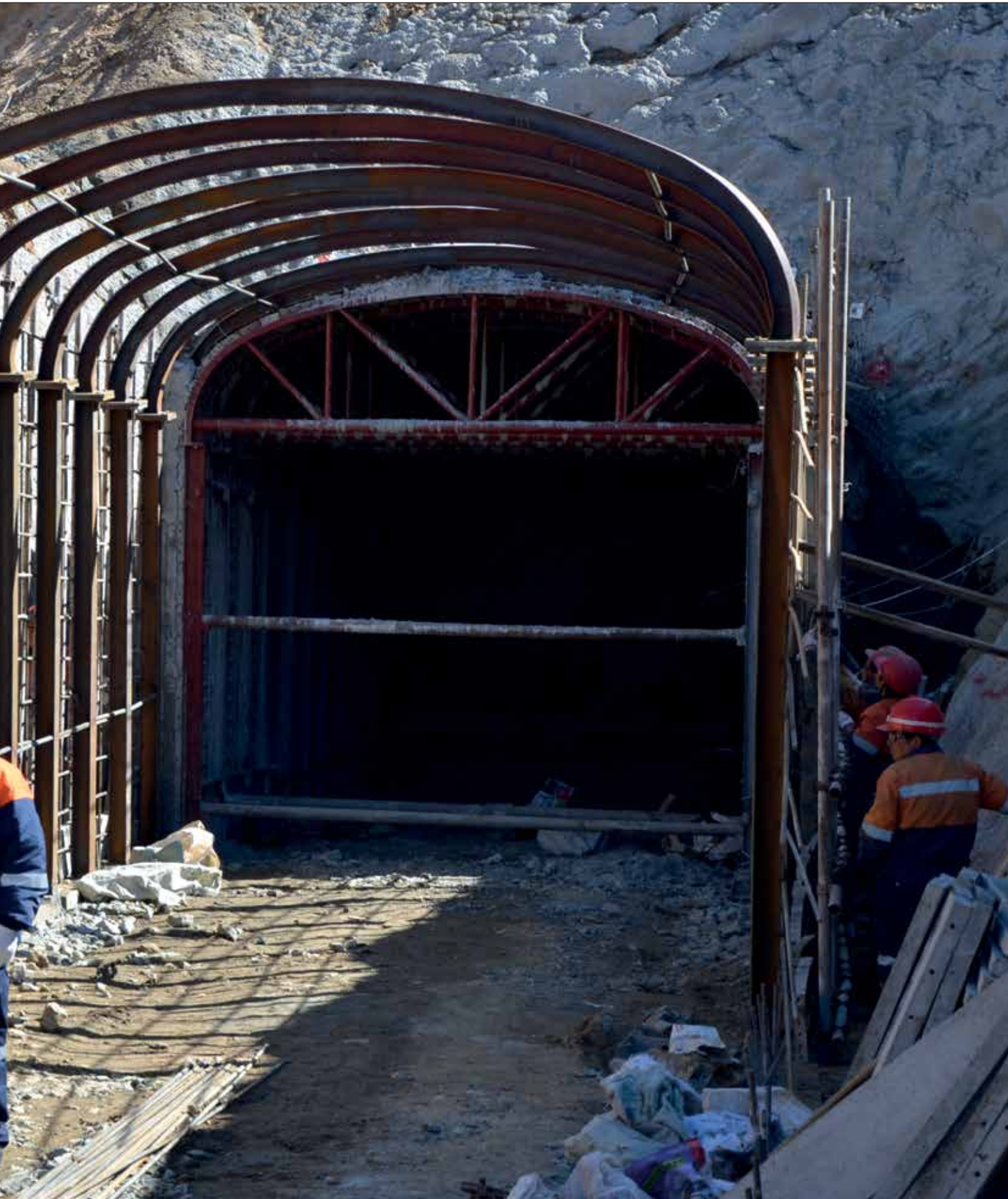
From left to right directors Adam Usdan, Roger Goodwin, Mladen Ninkov (Chairman), Rupert Crowe and Dal Brynelsen at the new second portal under construction at the Caijiaying Mine 23
