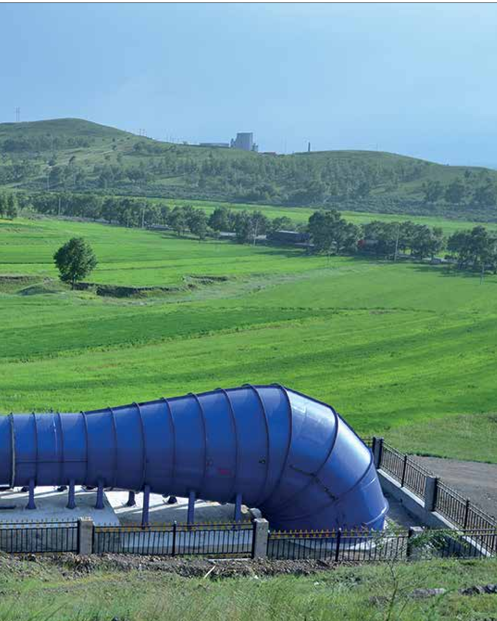
New North Ventilation Shaft with Caijiying Mine Site in distance providing perspective of Zone III 25
