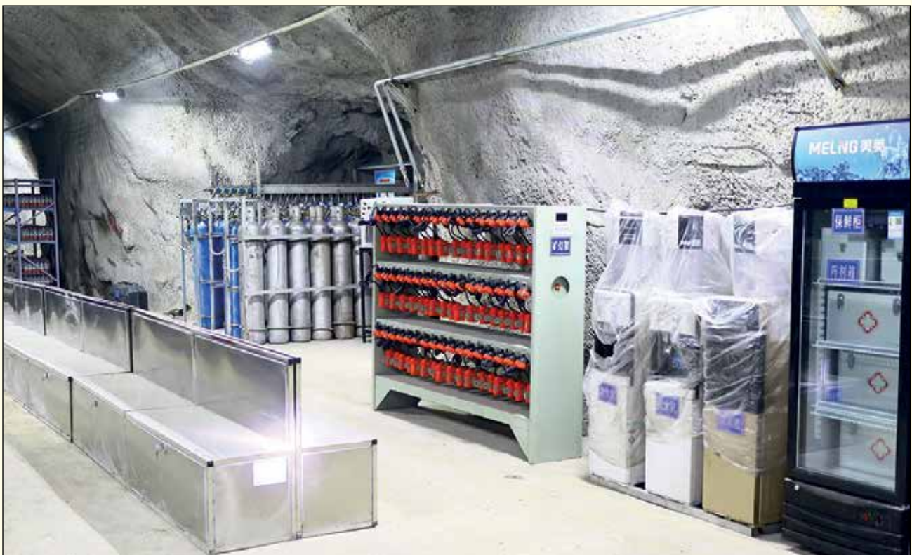
Underground Refuge Chamber at the Caijiaying Mine 1000m RL for 100 personnel
