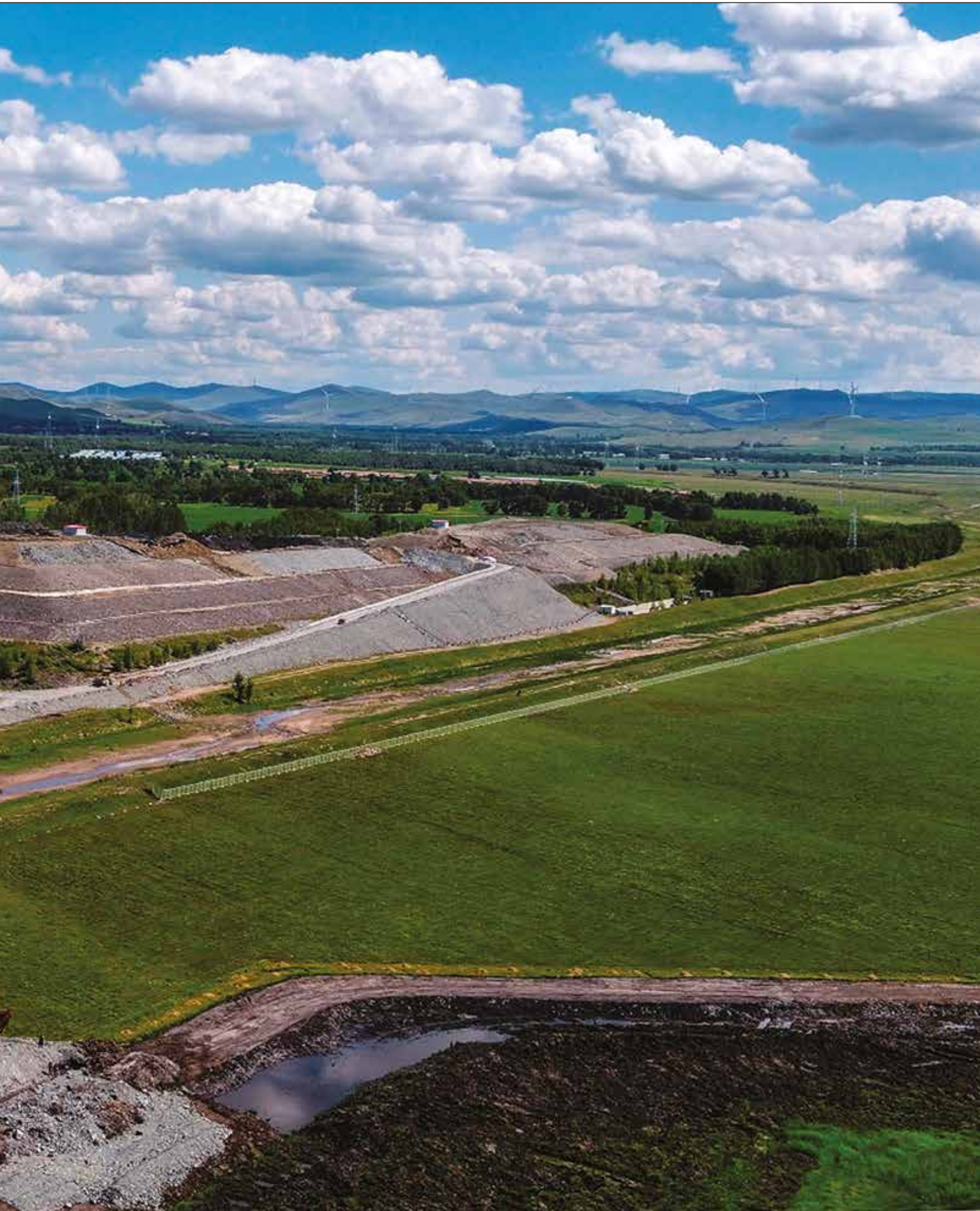
Tailings Facility Three in the background, with the new access road and bridge to Tailings Facility Four under construction 83
