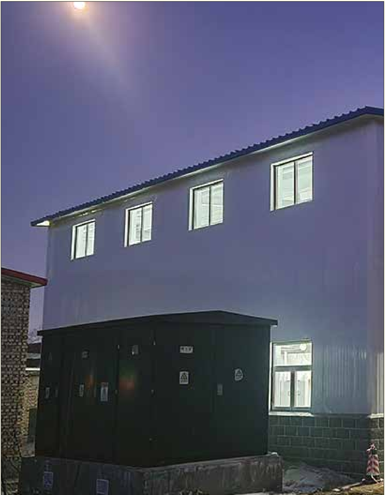
New Camp Electric Boiler
