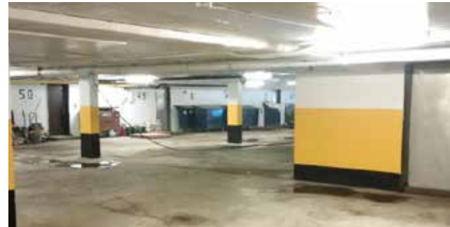
Francois Rive Verdun, Quebec City – Parkade restoration – Before
