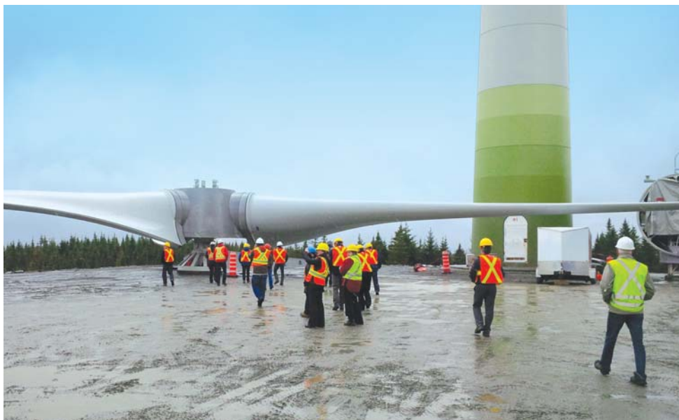
Crews prepare turbine blades during the construction of the Saint-Philémon wind facility in November 2014.
