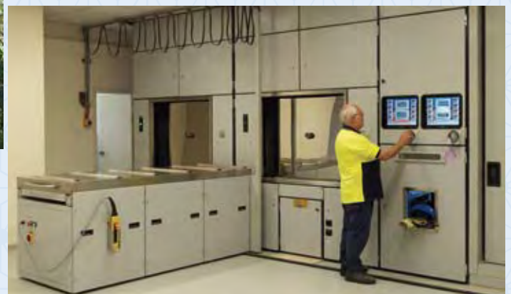
..... A recently installed cremator at Pinegrove Memorial Park.
