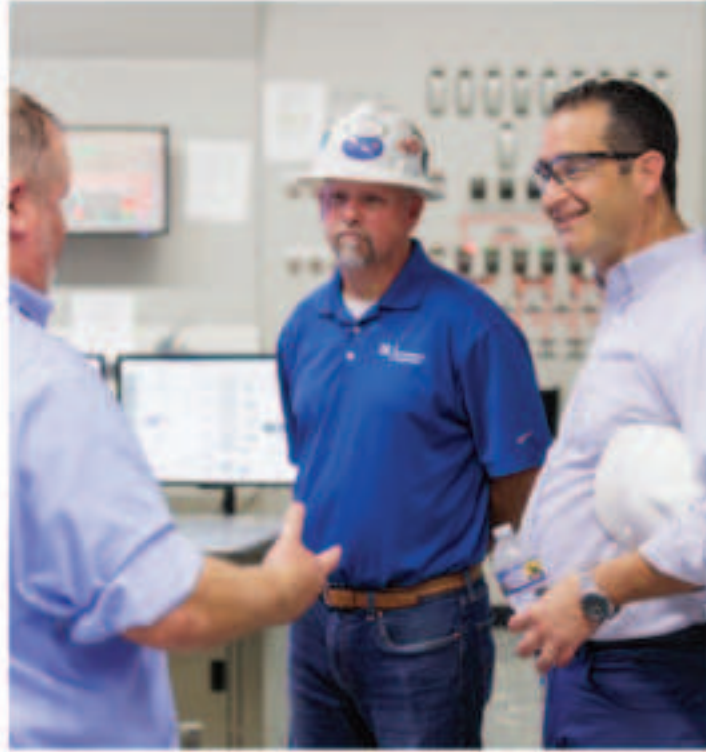
From left: Cumberland Fossil Plant operations manager Bobby Morgan and maintenance manager Chris Adams meet with TVA Chief Operating Officer Don Moul.
