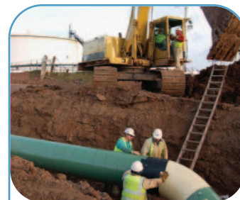
Construction continued in the United States on the Terrace Phase III expansion, expected to be in service in 2003.
