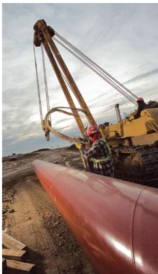
Alberta Clipper, which will provide Western Canadian producers additional transportation capacity to U.S. and Canadian markets, involves the construction of a new 914-millimetre (36-inch) diameter, 1,607-kilometre (1,000-mile) crude oil pipeline from Hardisty, Alberta, to Superior, Wisconsin.
