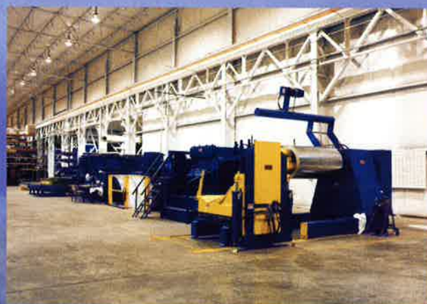
Roll metal uncoiler in new North building.
