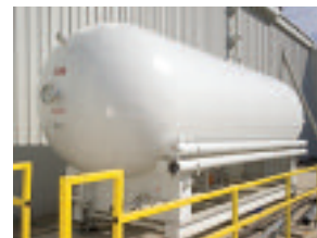
AAON has spent significant dollars installing new high-pressure storage tanks to accommodate R-410A.
