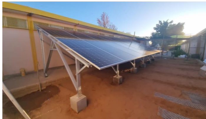
PV system installed at a school
