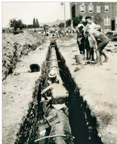
Plumber wiping joint where service was cut so as to make room for 20" supply main. August 28, 1898.
