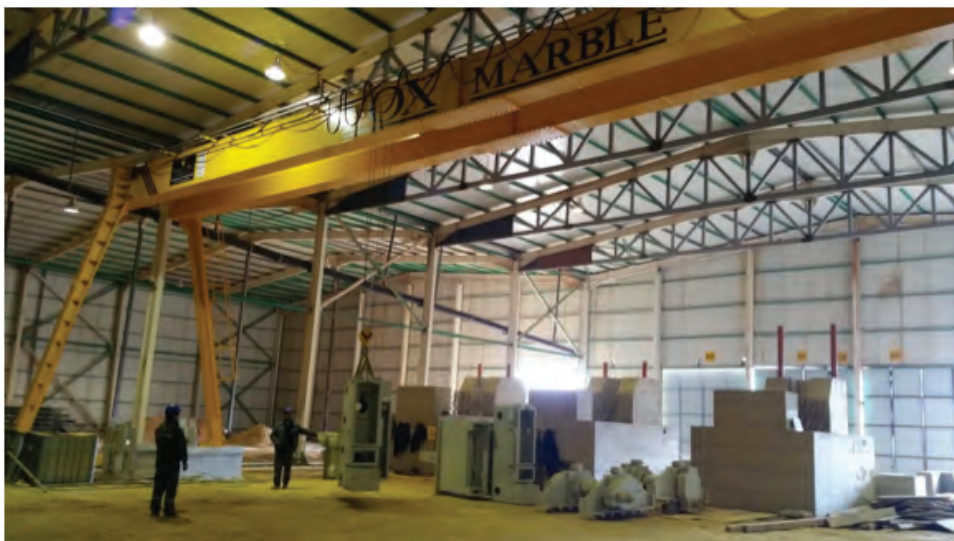
Internal gantry crane in operation
