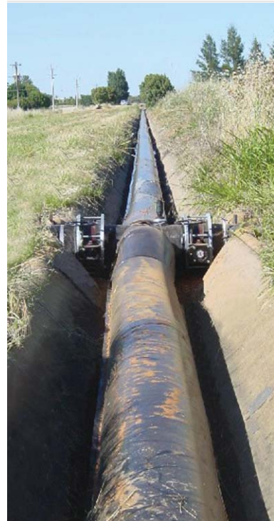
Channel liner water conservation
