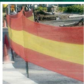
Barrier safety fencing
