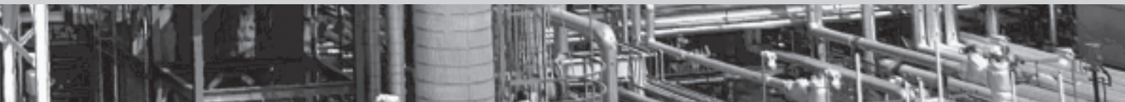
Calumet Shreveport Refinery; Shreveport, LA
