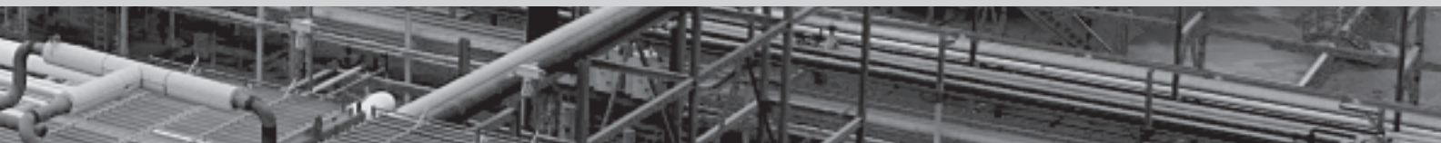
Calumet Shreveport Refinery; Shreveport, LA
