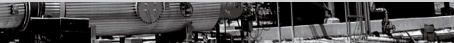
Calumet Shreveport Refinery; Shreveport, LA
