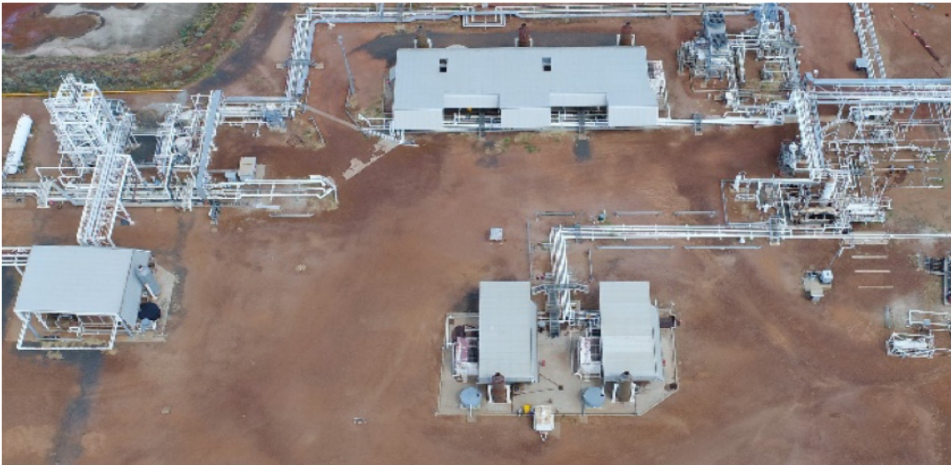
FIGURE 4 Kincora Gas Plant
