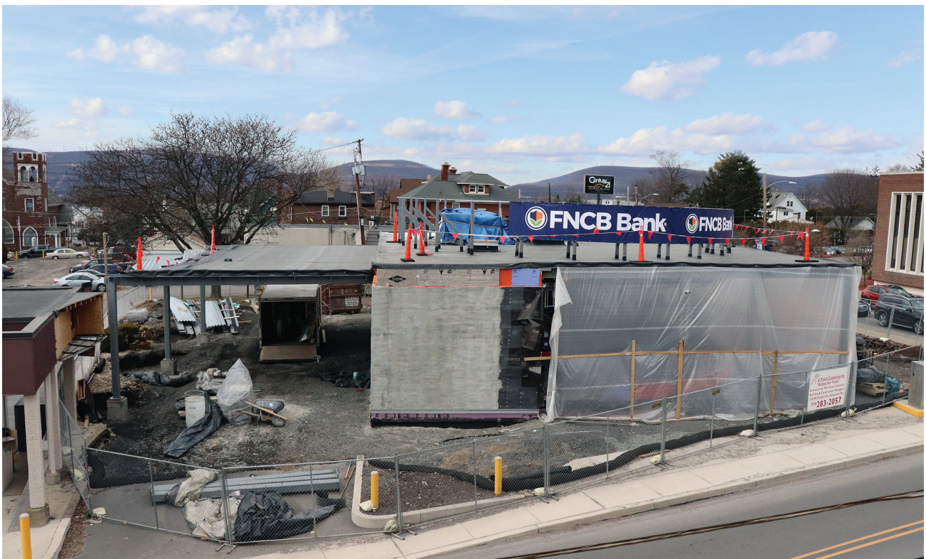
Construction is underway on FNCB Bank's new Main Office at 100 South Blakely Street, Dunmore. The current Main Office at 102 East Drinker Street, will relocate to this new location when completed in the second quarter of 2019.
