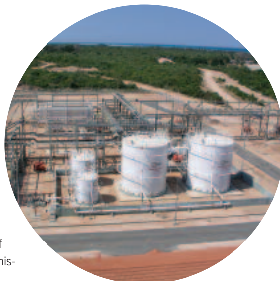
Two trains are used to process gas production from the Songo Songo field.
