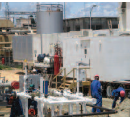
Top ↑ Orca employees installing a new power cable on the Songo Songo Gas Processing Plant.
