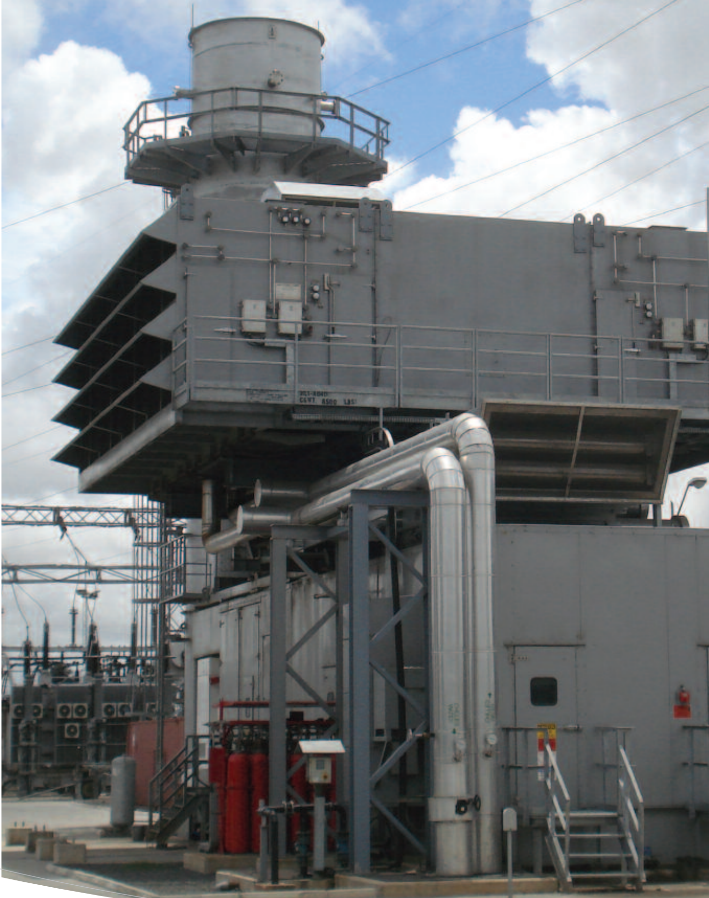
Above ↑ TANESCO'S Ubungu plant at Dar es Salaam produces electrical power from six units. Shown above is UGT6, the most recent addition to the plant. 19.5% of the natural gas used at Ubungu is Additional Gas supplied by Orca Exploration.
