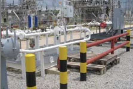
LEFT Over 2007 Orca increased the capacity of its low-pressure gas distribution system by adding a second pressure reduction station.
