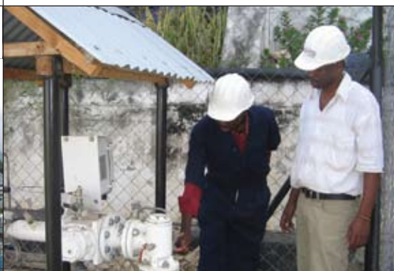
Orca made further upgrades to its low pressure distribution system in 2007 and now serves 17 industrial customers in the Dar es Salaam area.
