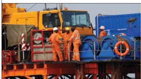
Remedial work on SS-9 has increased the estimated maximum flow rate from 20 Mmscf/d to 55 Mmscf/d.
