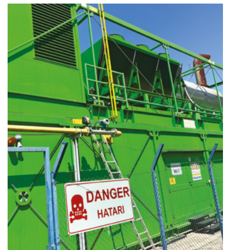
Gas Generator pipe inlet
