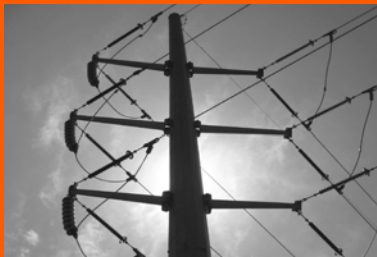
MEYER UTILITY STRUCTURES
