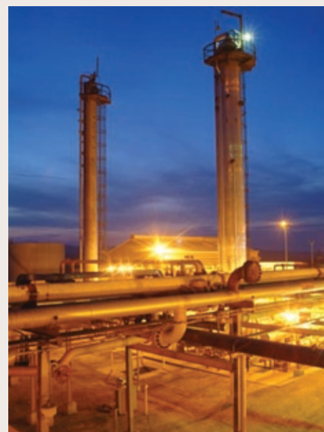
Inergy's natural gas liquids (NGL) business located in Southern California near Bakersfield is just completing a major expansion project expected to be operational by February 2009.
