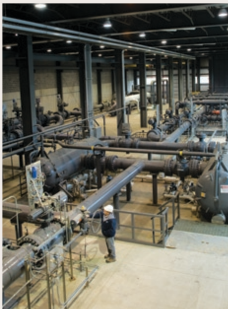
Inergy's Stagecoach facility is a state-of-the-art, multi-cycle natural gas storage operation located in Tioga County, New York. It is the core of Inergy's gas storage infrastructure in the Northeast.
