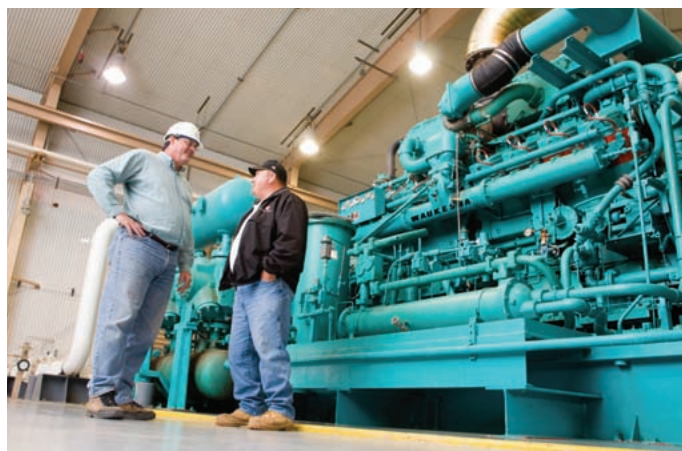
Inergy's Steuben natural gas storage facility currently has 6.2 Bcf of working gas storage capacity. Here two employees discuss operations in front of the compressor unit.
