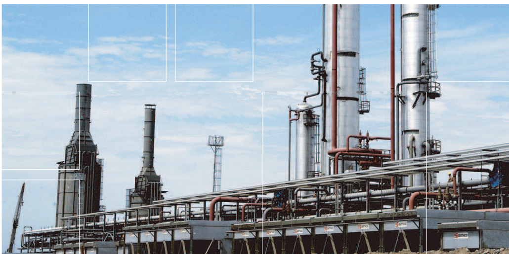
Pisco Gas Fractioning Plant for Camisea
