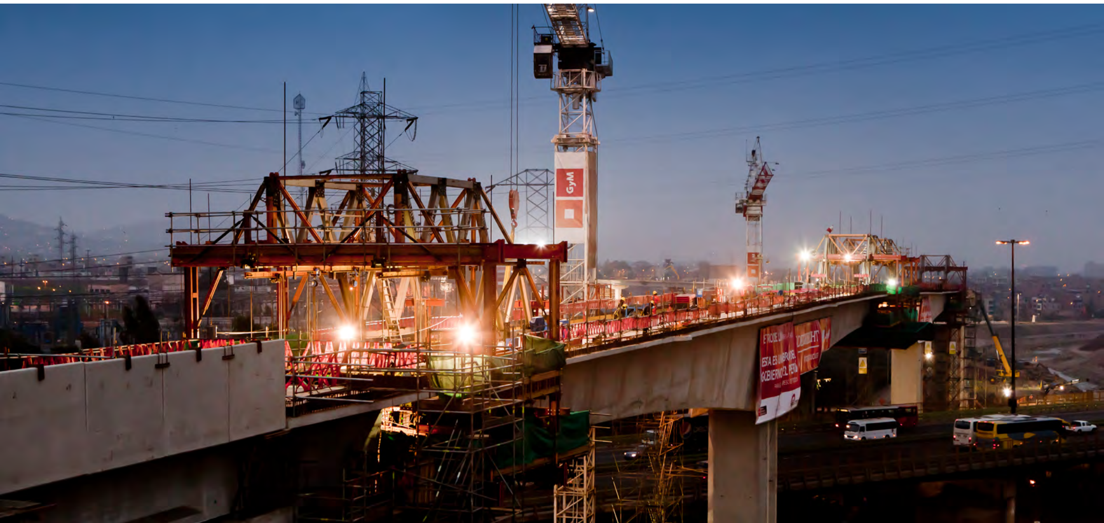
▲ Construction of The Lima Metro, Line 1 Section 2. (Grau Ave. – San Juan de Lurigancho)
