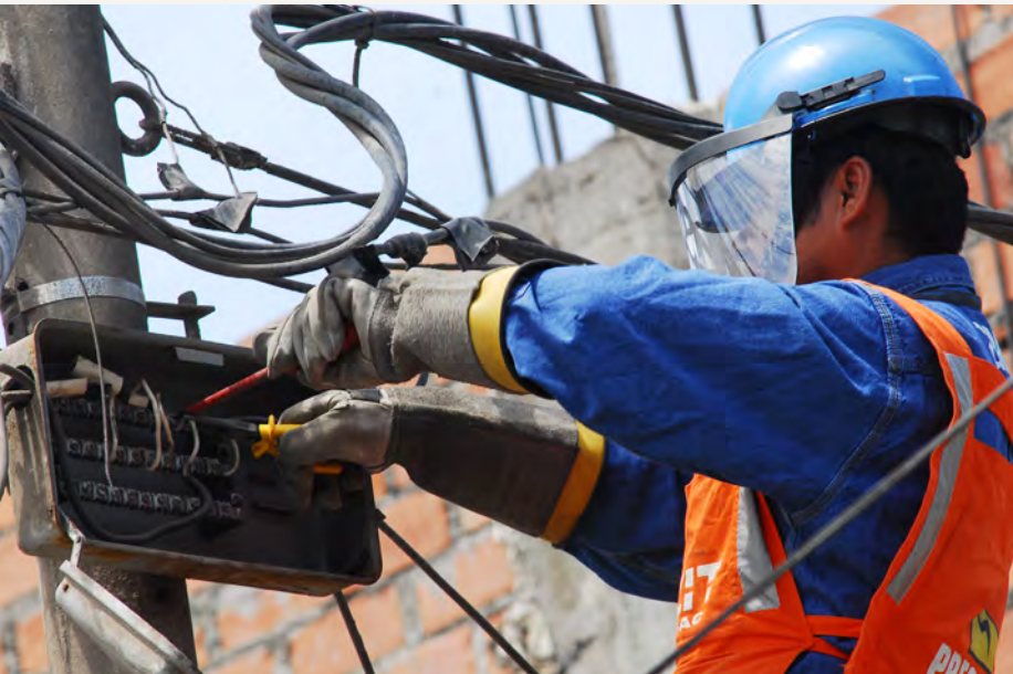
▲ Technical and commercial operations in medium and low tension
