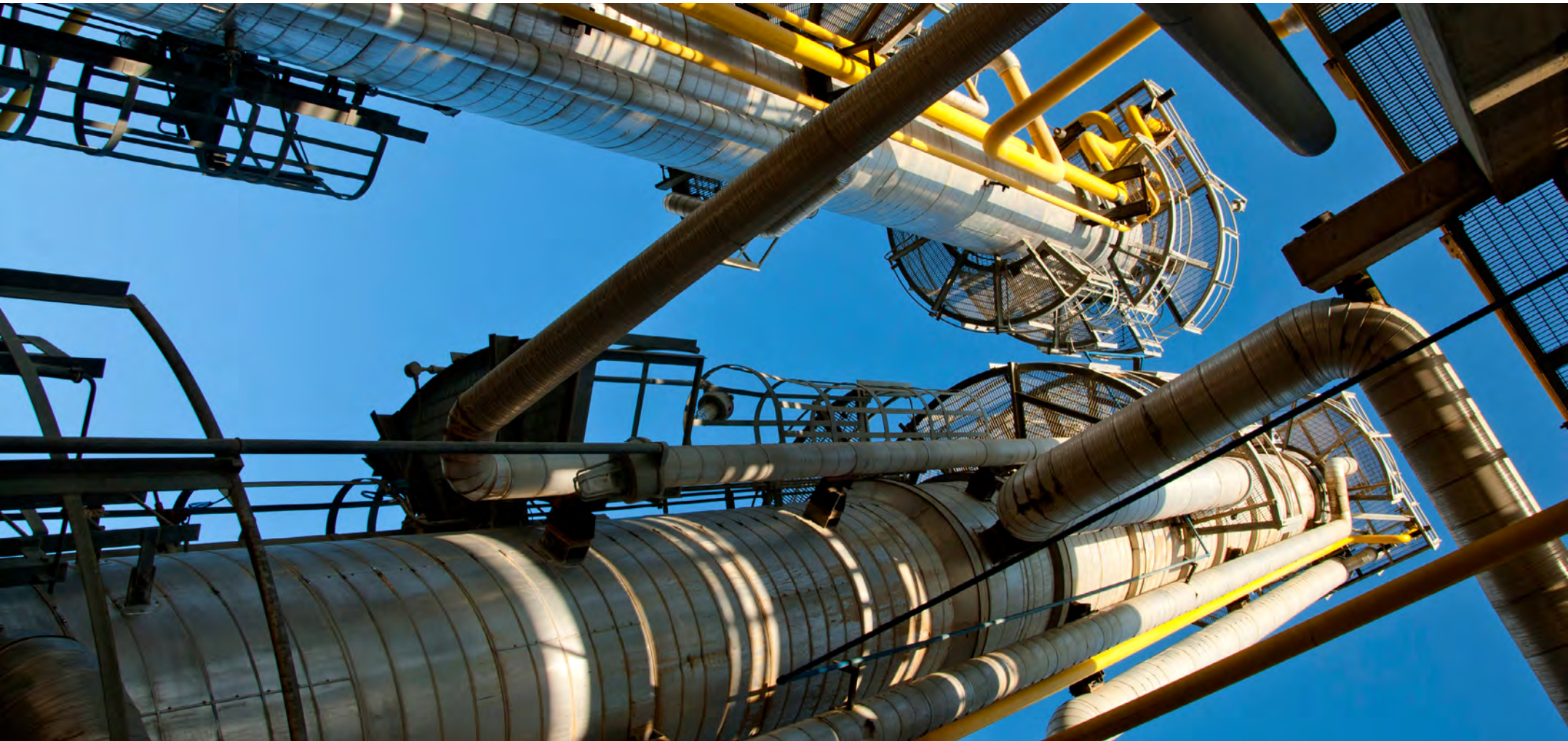
▲ Talara Gas plant
