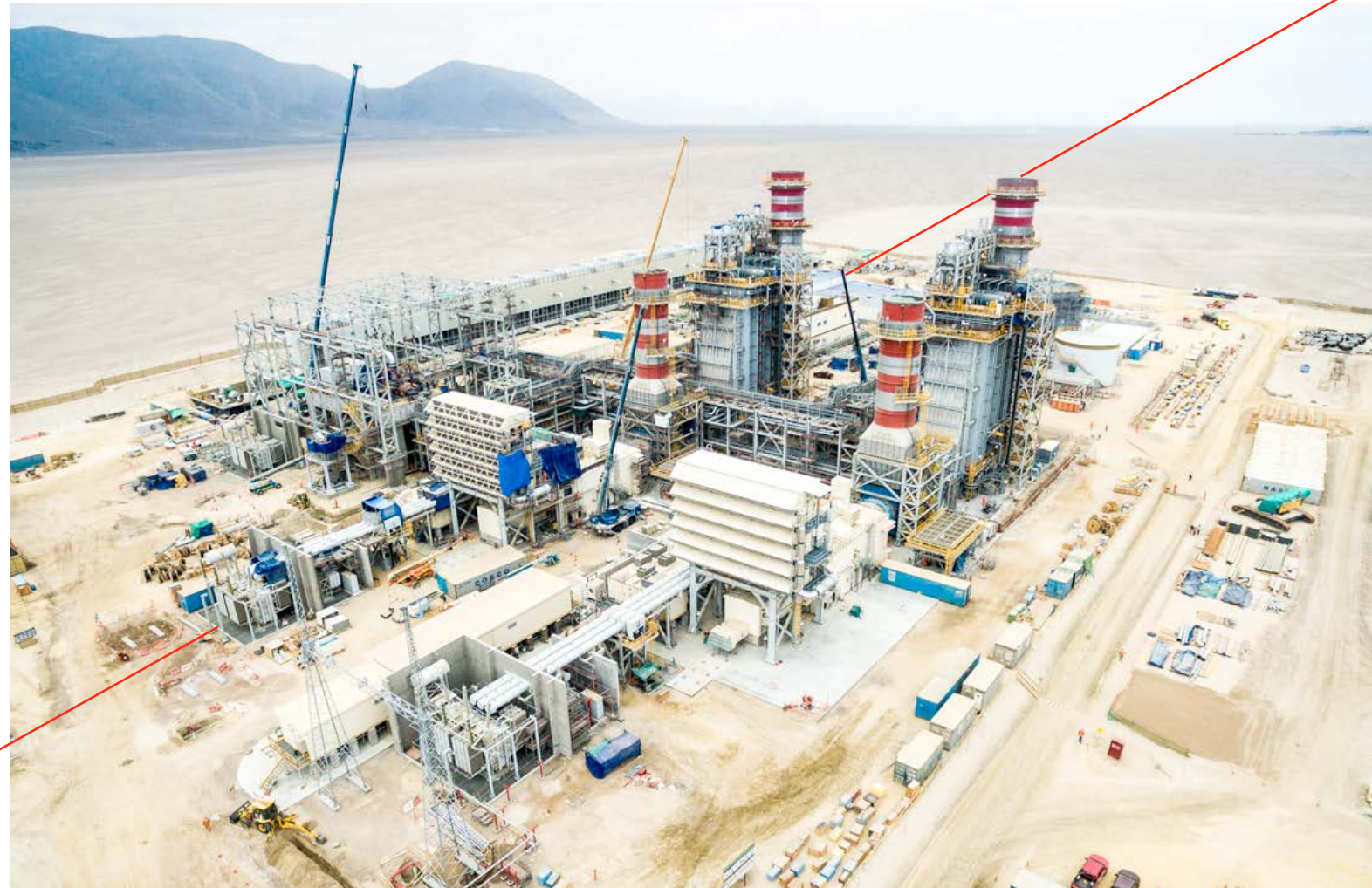
» Kelar Combined Cycle Power Plant Mejillones, Chile
