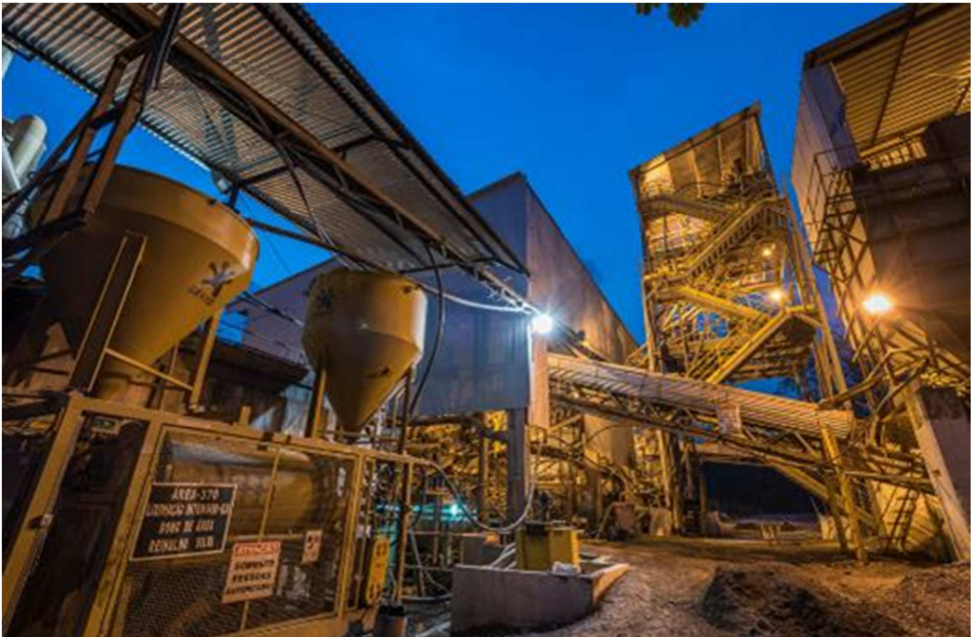
Figure 4- The Palito Complex process plant
