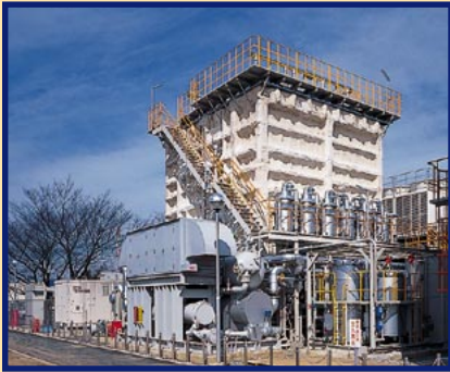
A super-cogeneration system at the company's Fuchu Operations fuses a gas-turbine cogeneration system with an ice heat storage system that uses inexpensive nighttime power.
