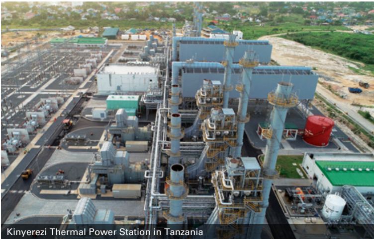
Kinyerezi Thermal Power Station in Tanzania
