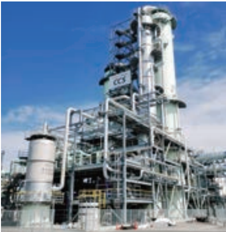
Large-scale carbon capture facility
