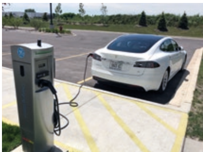
Electric car charging point at the new headquarters building for Renishaw, Inc.
