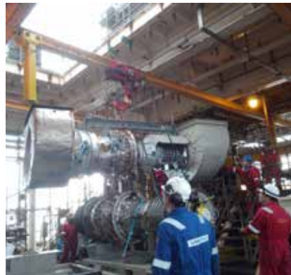
Improving core equipment with changeout of Bruce's LPBC 9-tonne gas turbine
