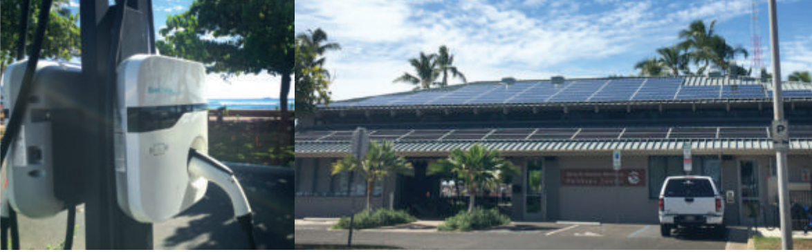
Above: The Pacific Current rooftop solar system and EverCharge EV charging station power the Harry and Jeanette Weinberg Ho'okupu Center while encouraging EV adoption.
