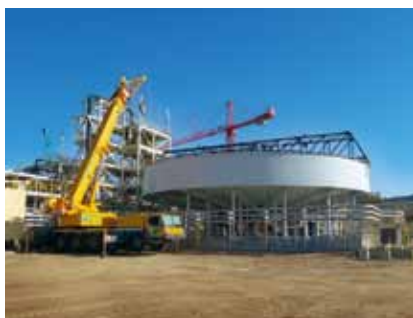
New thickener at the process plant
