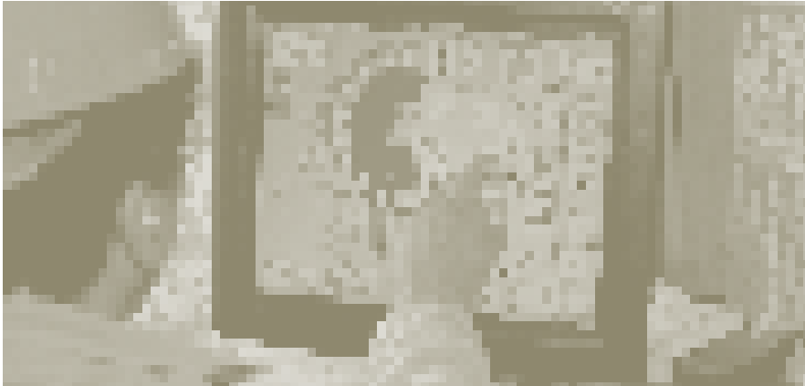
Ilo Smelter - Anodes plant, control panel - Peru
