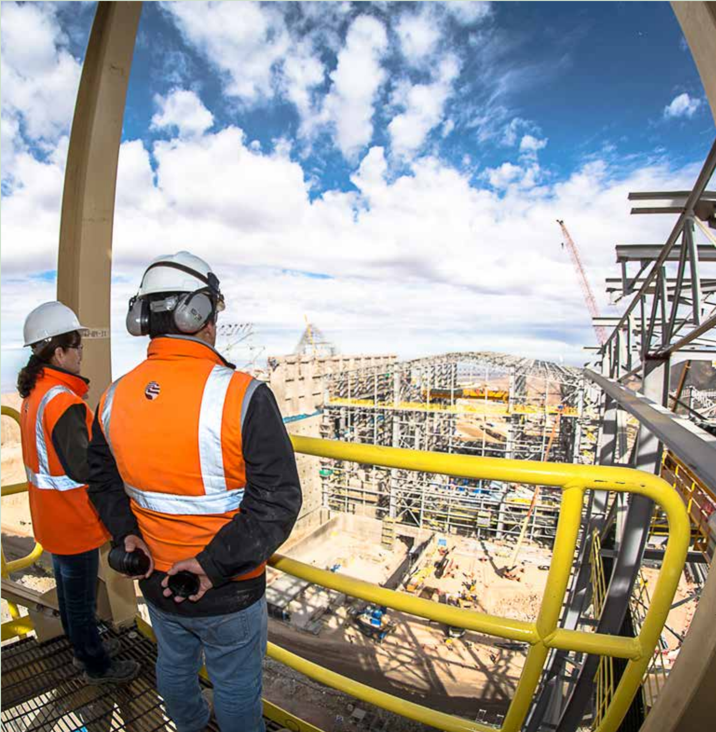
View from the new HPGR plant in the Toquepala Concentrator, Tacna, Peru.
