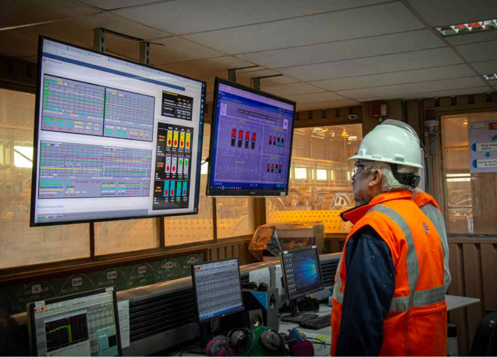
// Control center, Cujane Concentrator, Peru
