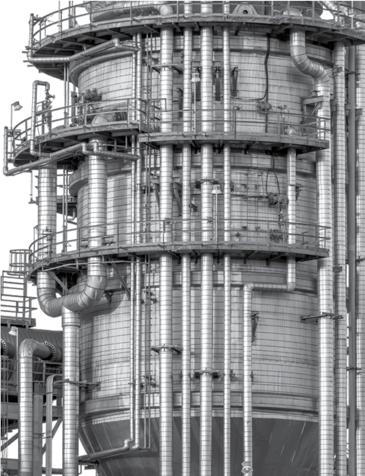
| Wood River Refinery Distilling North Vacuum Tower ROXANA, IL
