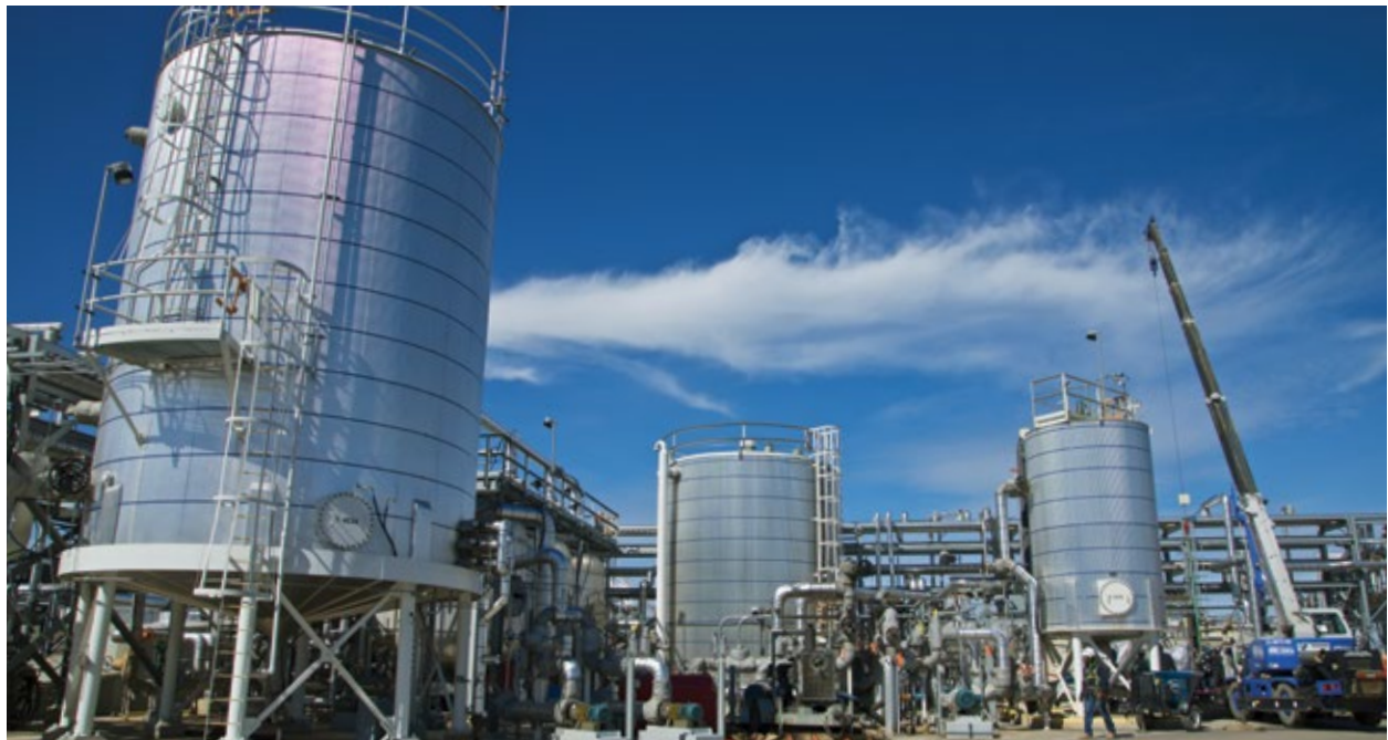
Billings Refinery Water Treatment Facility BILLINGS, MT
