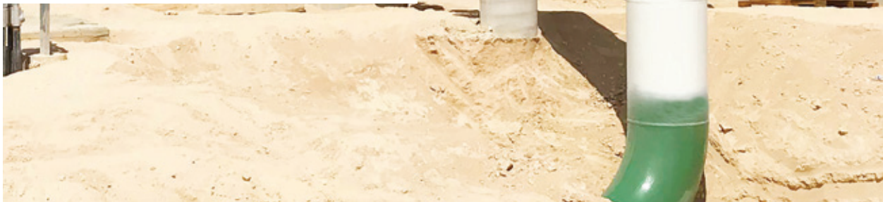
La Pryor Storage Terminal Gray Oak Pipeline LA PRYOR, TX
