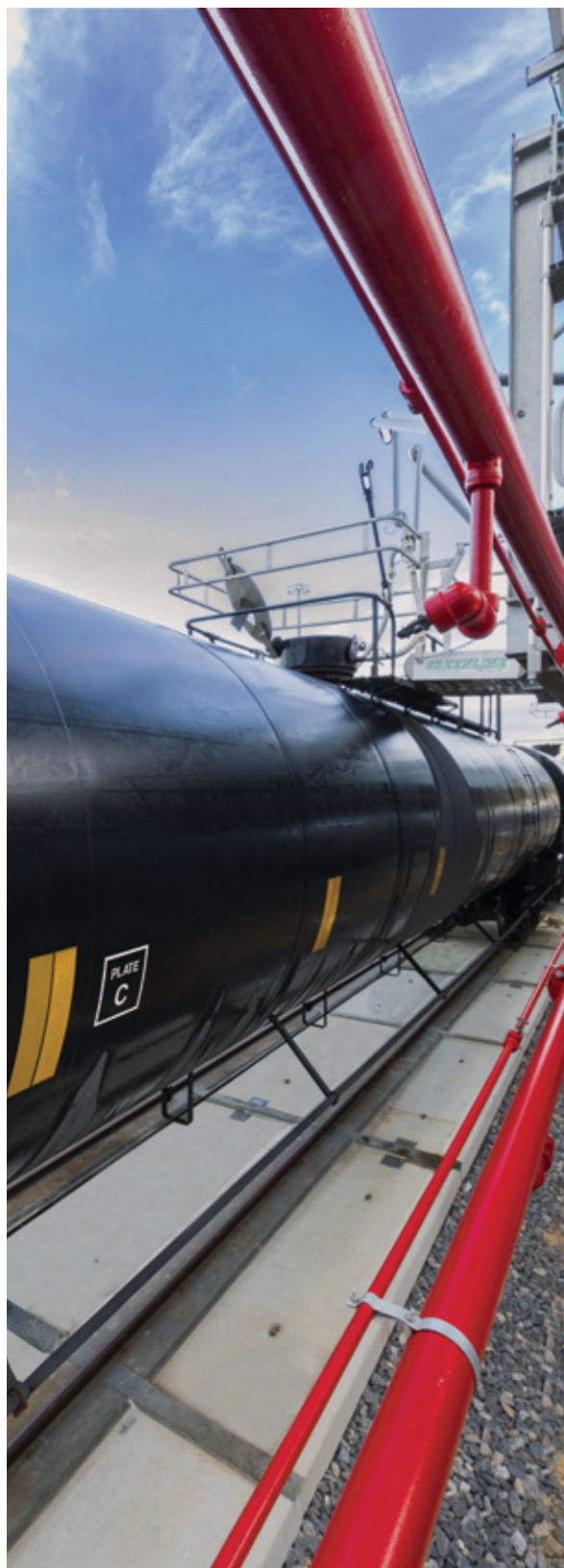
CPChem Rail Car Area OLD OCEAN, TX
