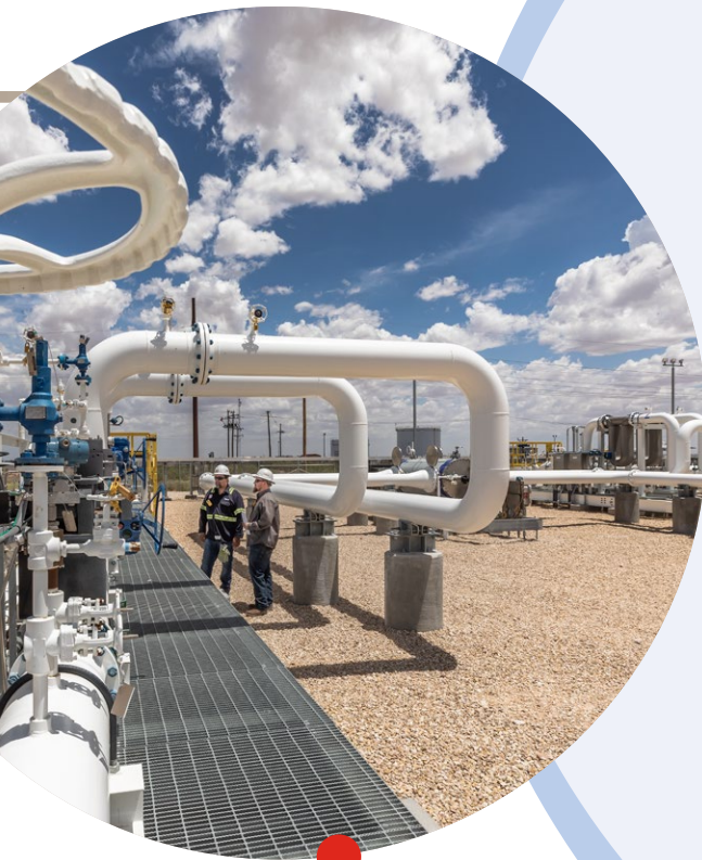
Gray Oak Pipeline Wink Facility WINK, TX
