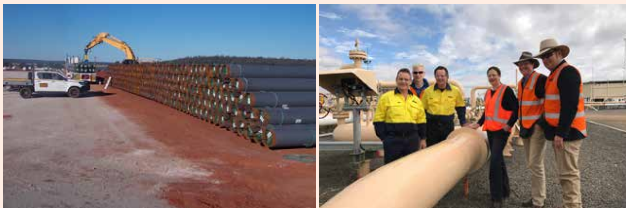
From delivery of pipes in November 2016, to the official opening in June 2018, the Reedy Creek Wallumbilla Pipeline is already providing commercial options for APLNG to move its gas
