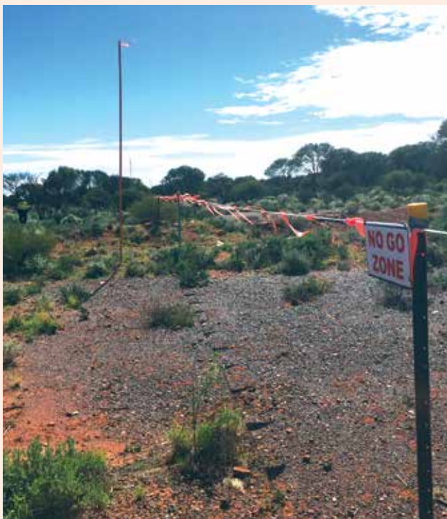
Bunting boundary protecting Yamarna cultural heritage site during construction of the Yamarna Gas Pipeline, Western Australia
