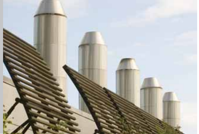
Crown Melbourne, Cogeneration plant standby boilers
