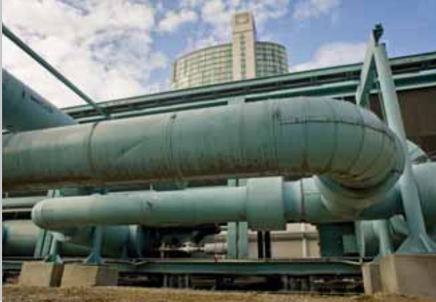
Crown Melbourne, Cogeneration plant rooftop equipment
