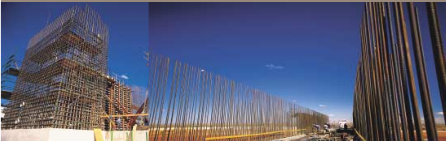
L to R: Construction of Sag Mill Train 2 Pedestal and Reclaim Tunnel Train 2 – Telfer
