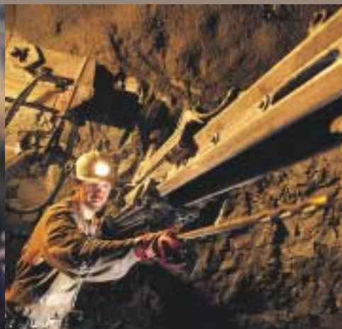
Brett Vaughan, underground miner, fitting a rock bolt into the boom of an underground drill prior to installation
