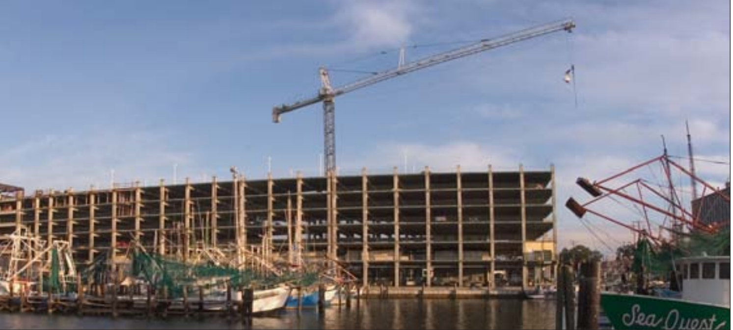
Shrimp boats at the dock behind the rising Hard Rock Casino under construction symbolize the past and the future of the Mississippi Gulf Coast and The Peoples Bank.
