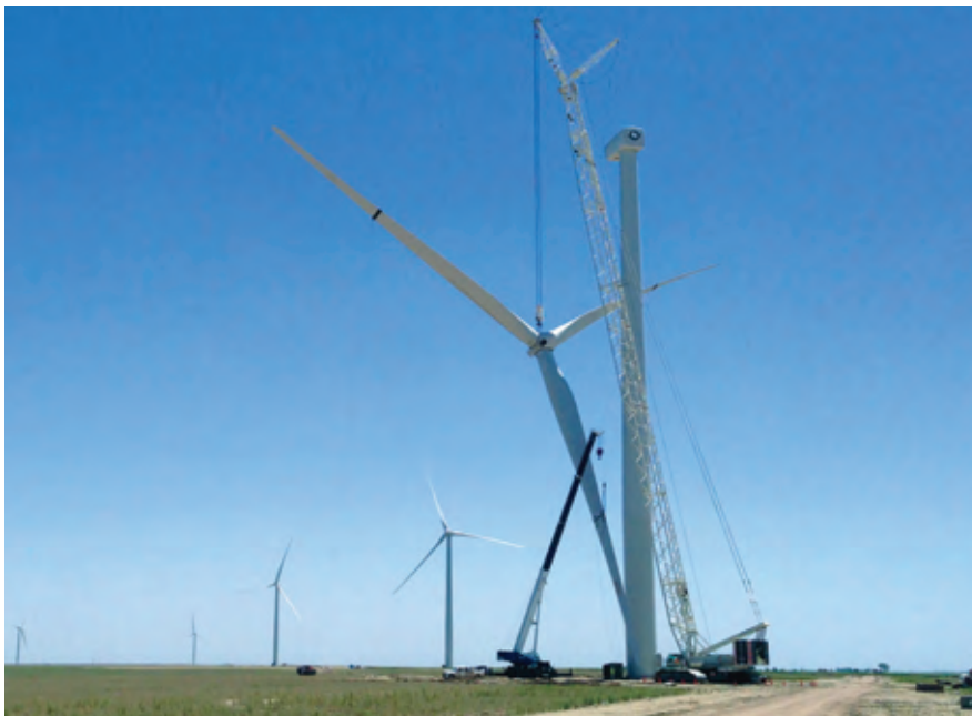
NextEra Energy Resources' Limon III Wind Energy Center, Lincoln County, Colo.
