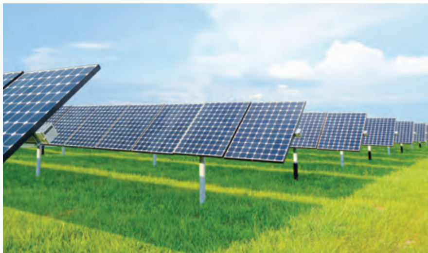
FPL's DeSoto Next Generation Solar Energy Center, DeSoto County, Fla.
